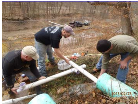
MCWA members installing piping to divert mine water discharge to micro-hydro turbine
