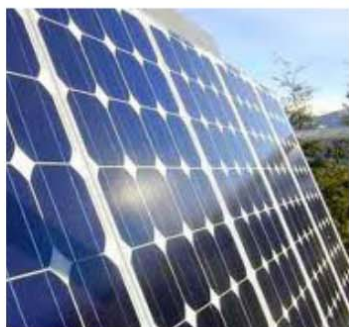
Detail of south facing solar array
