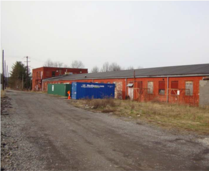
Above photo showing rear of Corbins building, which will be “deconstructed” to salvage structural materials.
