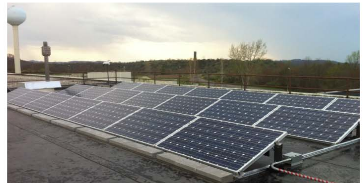
Above photo shows the awning-style solar panel array installed at University High School
