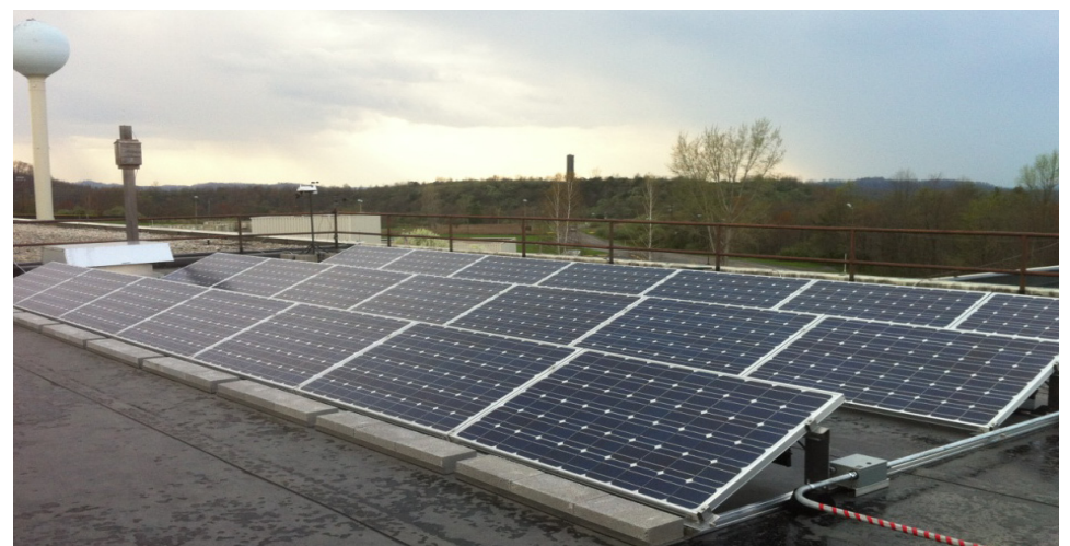
Above photo shows the awning-style solar panel array installed at University High School
